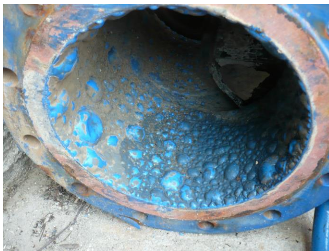
Figure 4. - The iron fitting used for thermal water pipeline
