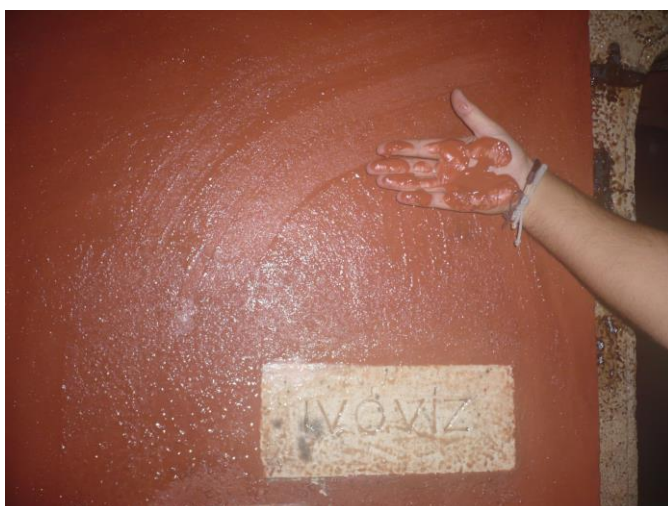
Figure 3. - The wall (with turkish mortar) after thermal water attack
