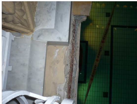
Figure 1. - Corrosion of the steel reinforcement in concrete
